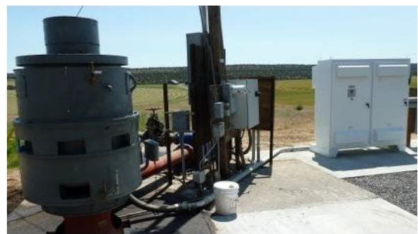
Figure 2. Variable Frequency Drive-Controlled Pump (Photo: USDA)
