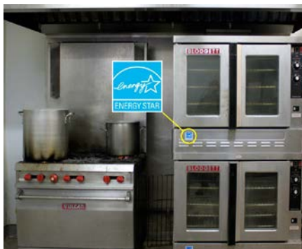
Figure 1. ENERGY STAR ovens
