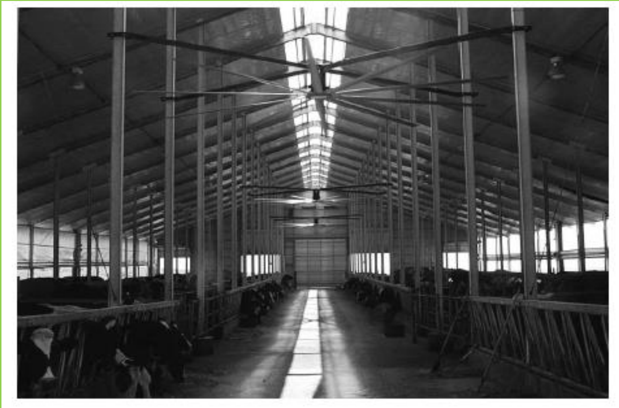
HVLS fans in a freestall barn
