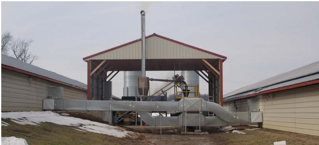
Figure 2. The Global Re-Fuel system at the Rohrer farm is located between two poultry houses to reduce length of ductwork.
