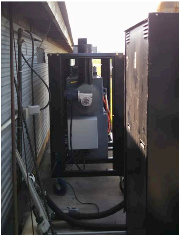
Figure 4. This is the wet scrubber before it was connected to the exhaust of the combustion unit.
