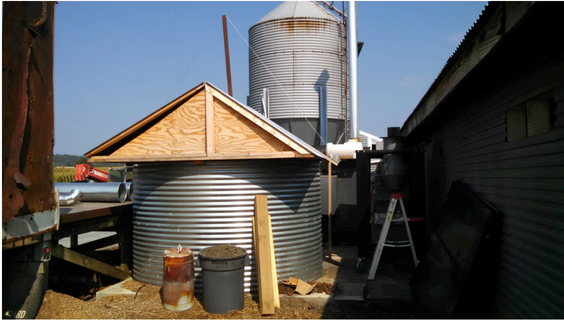
Figure 1. The silver cylinder with the wooden “A” frame cover is the litter storage hopper. It has a sweep arm that feeds the litter into an auger that meters the litter into the combustion chamber.
