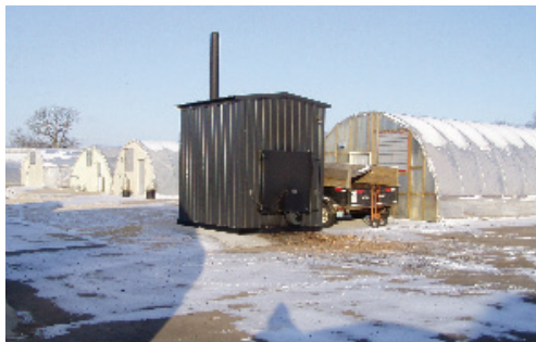
Figure 1. Outdoor wood-fired boilers can be centrally located on a site. Many are suited for the elements and do not require the protection of a building or shelter.
