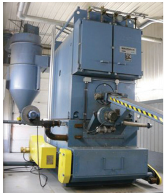
Figure 3. This wood-chip boiler's fully automated stoking system significantly reduces the daily labor required to maintain the system.
