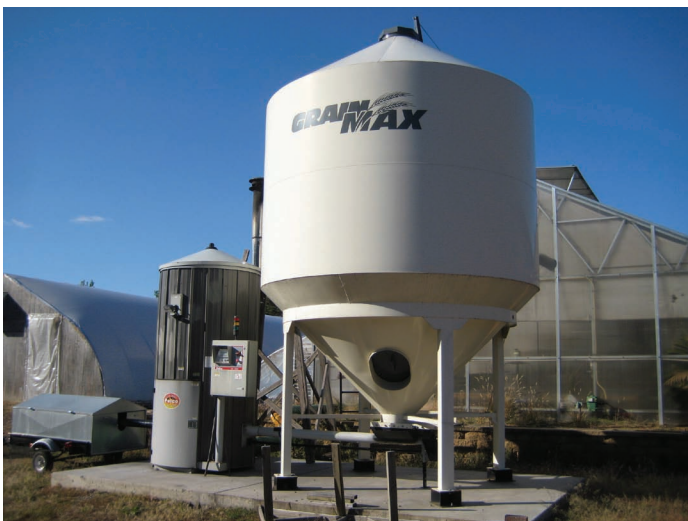
Figure 4. This commercial-sized pellet boiler is equipped with a storage bin and an ash cart, part of the automatic ash removal system.
